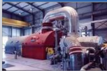
Steam Turbine Generators
