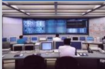
Instrumentation & Control Systems
